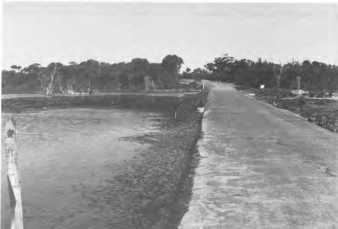
The flow of saline water from Yenyening Lakes into the Avon River is presently controlled by flood gates
