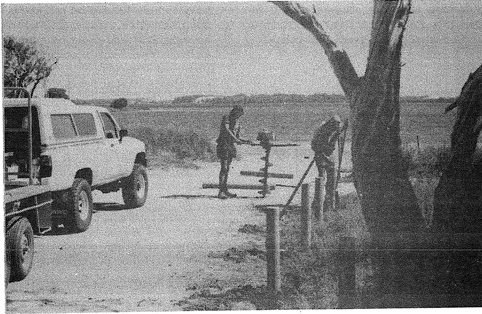
Barriers are required to restrict vehicle access to foreshore areas.
