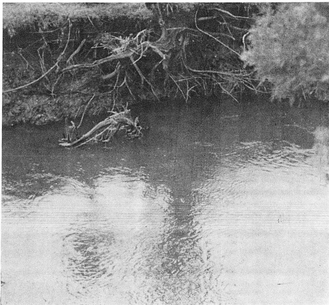
Plate 4: Sampling point F2 showing severe erosion of river bank.
