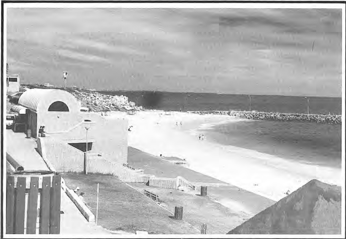
Photograph 7. Cottesloe main beach. The concrete wall on the foreshore side has been cracked by storm water action.
