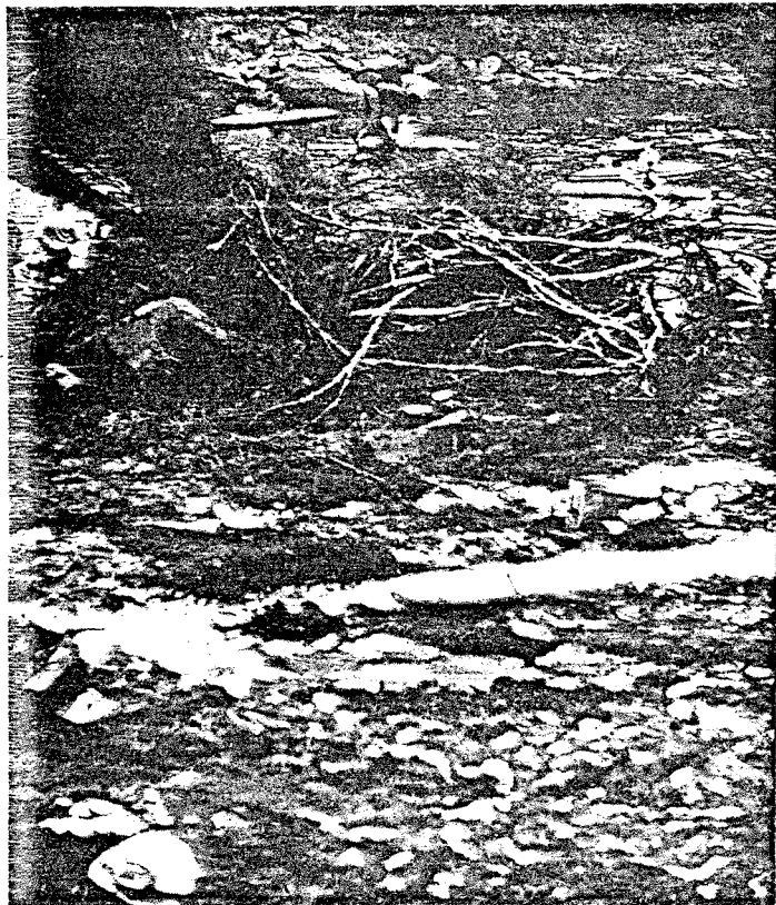
Fig. 16 : Following overnight rain, the clearing on Sunday morning was slippery and deep wheel ruts from the bulldozer collected water. Rubbish is evident in the foreground.
