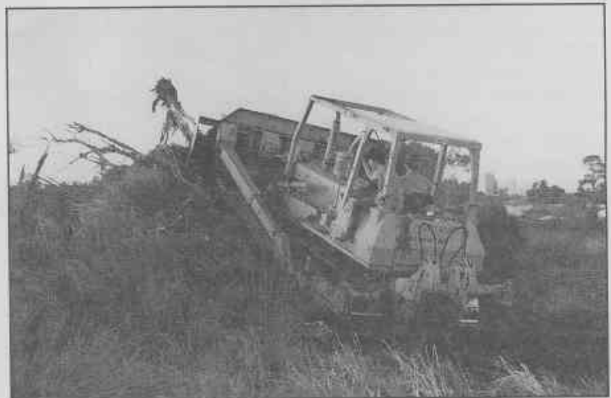
Julie and Greg in the cab of the D7 bulldozer, constructing the basin of the wetland (1988). Photo courtesy of Julie Bousfield.
