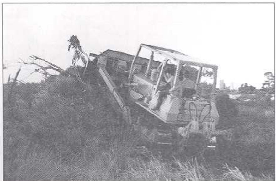
Julie and Greg in the cab of the D7 bulldozer, constructing the basin of the wetland (1988). Photo courtesy of Julie Bousfield.
