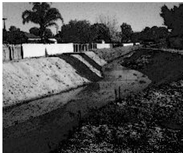
Paterson St Drain after earthworks to create meanders and lessen the slope of the bank. (Photo supplied by Rosemary Glass, BICM).
