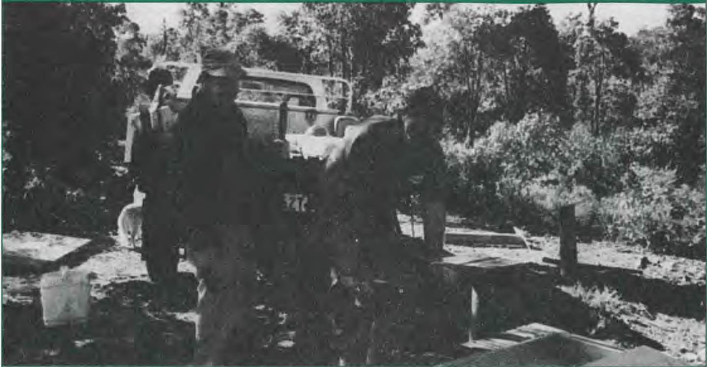
John Bowler and John Robertson installing a boot scrubber to prevent the spread of dieback in the Ellis Brook Reserve.
