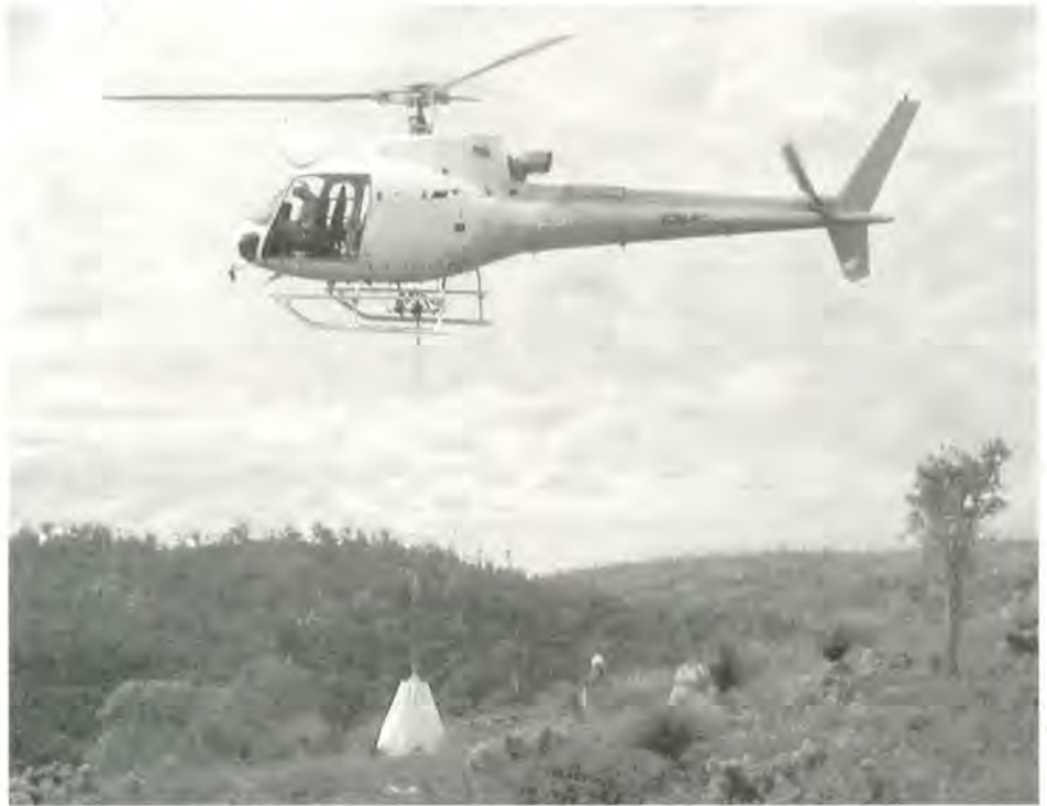
A helicopter places a large bag of roadbase where it is needed for the trail construction in Ellis Brook Valley. (Photo: John Bowler)
