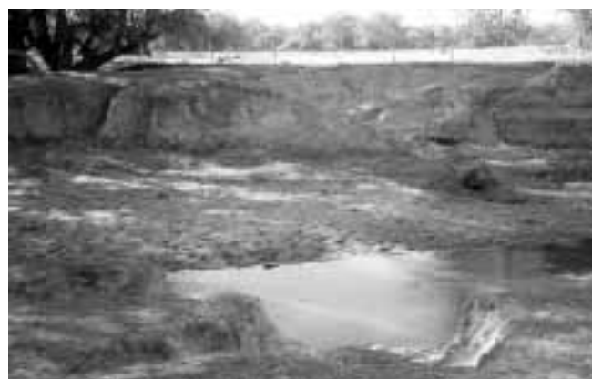
Figure 6. Dandalup River prior to installation of LWD. The site selected for one of the log riffles was severely degraded and destabilised due to cattle trampling.
