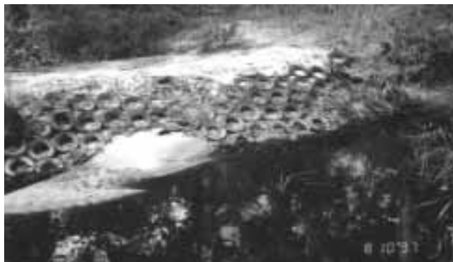
Figure 16. Sediment accumulation in car tyres placed to prevent bank erosion.
