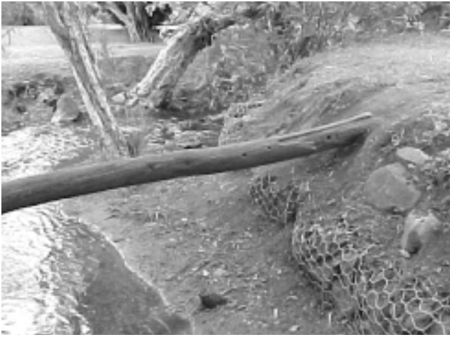
Figure 5. Gabions. This site is also on the Neerigen Brook in Armadale. It is very close to an historical Aboriginal camping ground and needed approval to install the rock gabions. The City of Armadale installed the gabions (to reduce erosion) under the supervision of the local Aboriginal community.
