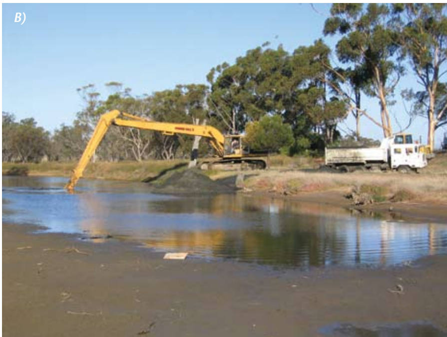
Figure 3 Depending on the site, a dredge (A) or a long-reach excavator (B) may be more suitable for extracting sediment
