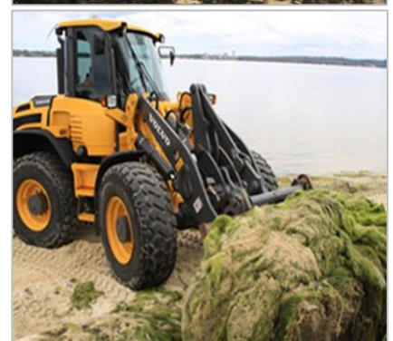
Photos: Submerged seagrass, Halophila ovalis beds (top); accumulated seagrass wrack (middle); and removal of macroalga wrack (bottom).
