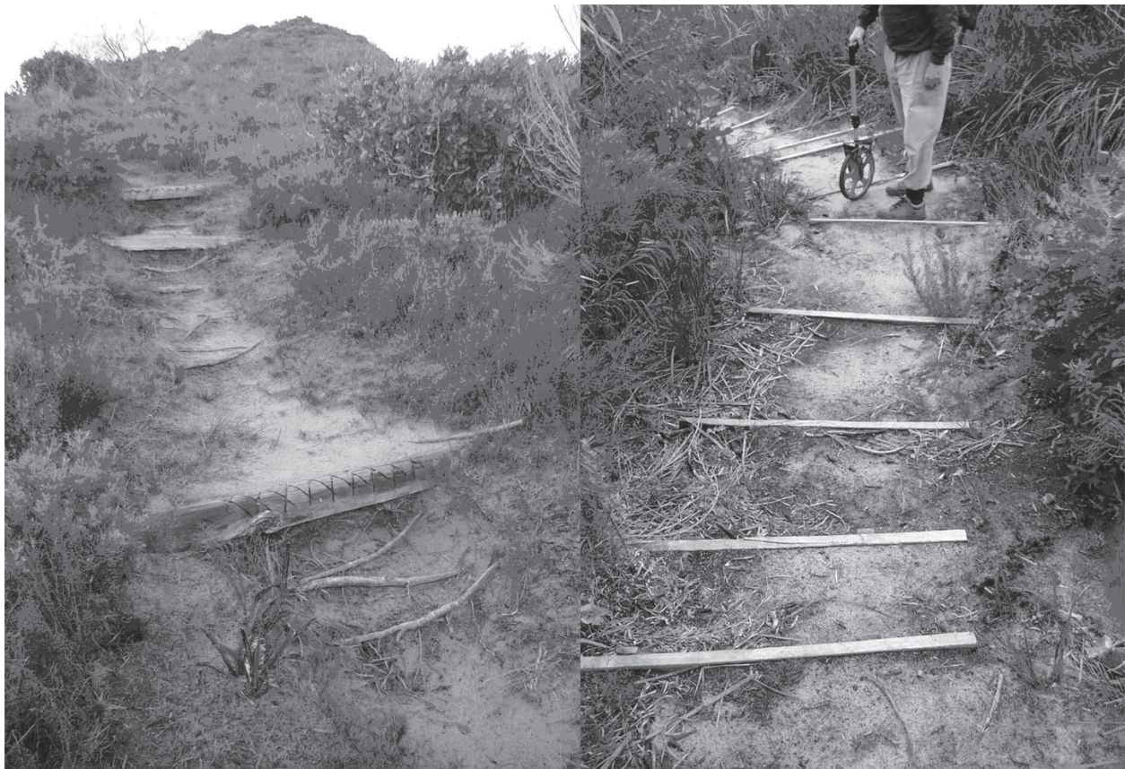
Figure 11. Water bars (left) with a tread space > 1m showing water erosion at the base of each bar due to the on trail waterfall created during surface water flow. Grouped steps (right) on a steep slope with a tread space of < 1m, show no signs of water erosion or soil movement. Bibbulmun Track in WCHNP
