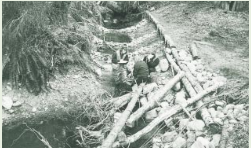
Photo 1: Wood and rock structures were placed in a tributary of the San Juan River, BC to create fish habitat and protect the banks. Flow is toward the bottom of the photo.
