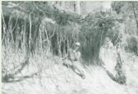
Scour of a stream bank leading to undercutting. Photo by Ian Rutherford.
