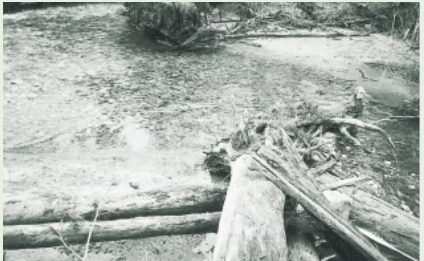
Photo 2: Log jam placed at bank in Lukwa Creek, BC to increase flow resistance, dissipate stream energy and reduce the likelihood of sediment wedge or nickpoint migration. Flow is from left to right.
