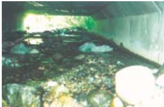
Left: Double barrel corrugated pipe culvert with baffle fishway Right: Large span box culvert with stream simulation fishway
