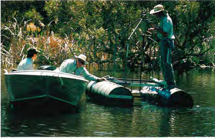
Figure 4: BOC Gases contractors installing dissolved oxygen probes for the automatic control system
