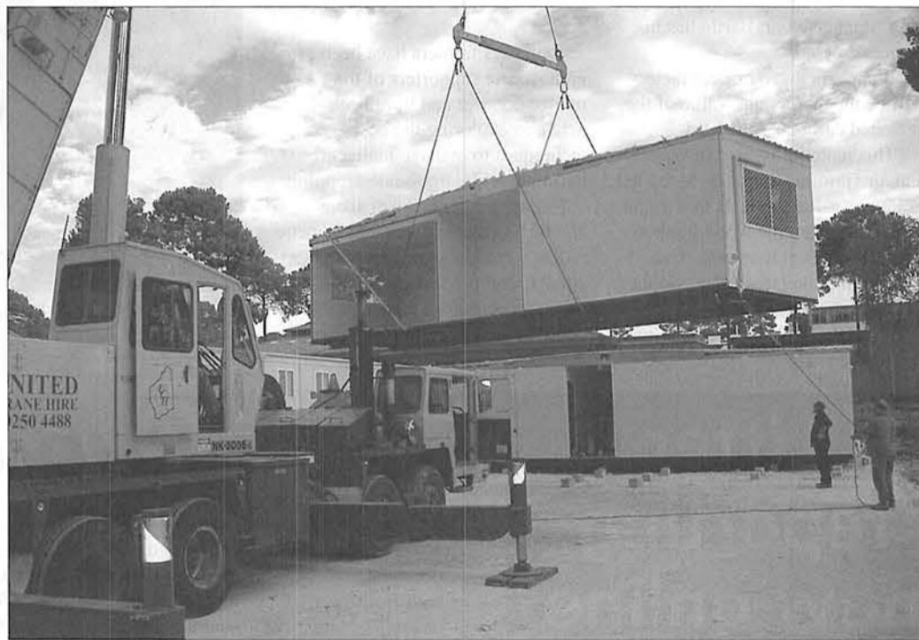
A section of the new demountable being lowered into place. Photo – Mark Neilson
