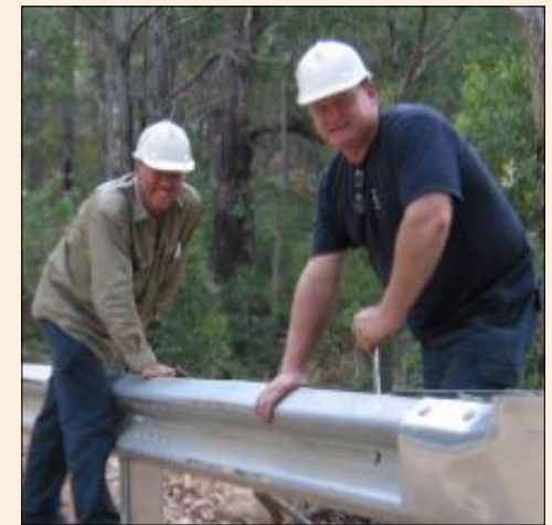
Overseers Geoff Styles and Phil Griffiths put the finishing touches on the Scarp Road bridge.
