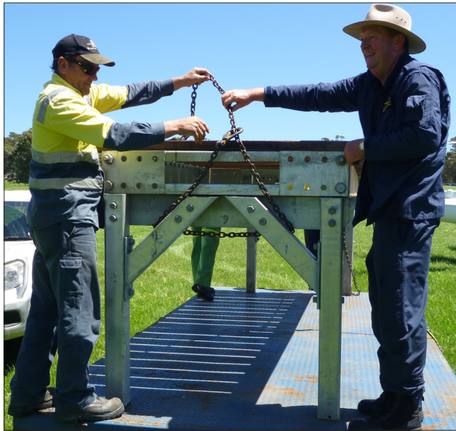
Graham White and pilot Dave Newman prepare the bridge to be air-lifted.
