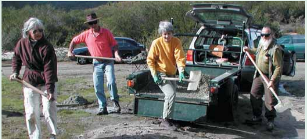
(From left) Heather Bowler, Rod and Rosemary Thompson and Marc Lane from the Friends of Ellis Brook Valley working to construct a settling pond. Photo – John Bowler
