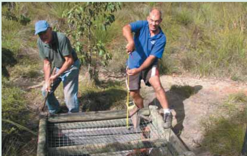
Ashley Rains (left) and Greg Hill repairing a well at Ambergate Reserve. Photo – Bernie Masters
