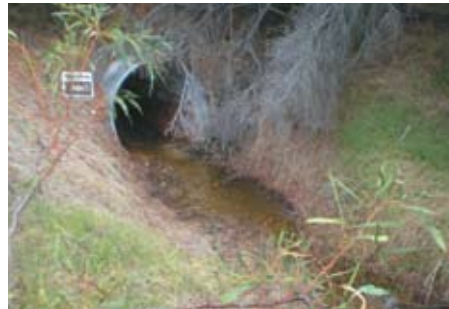
Despite south-west WA experiencing the driest year on record, recent high tides have resulted in rising groundwater inland from Mangles Bay. Photo – Hugo de Boorder
