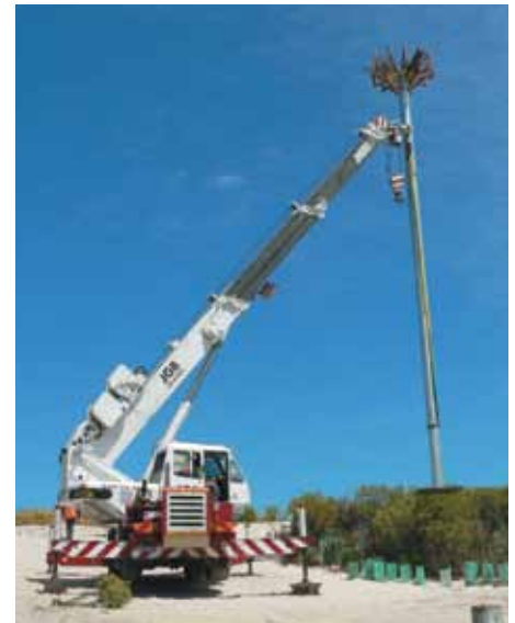
The erection of a 15 m osprey nesting pole at Coogee Beach involved two cranes and much wringing of hands but the outcome is impressive. The pole is being monitored by the community for any new arrivals. Photo – Steve Harwood
