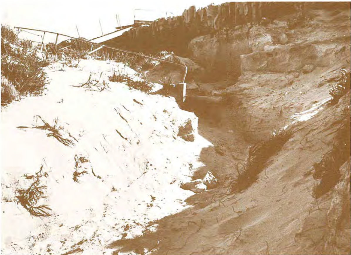
Photograph 15 Severe gully erosion caused by poor drainage control at Nine Mile Beach.
