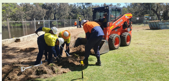
Above and below: Aboriginal trainees gaining practical experience for their Certificate II in Construction. Photo – CareyMC Pty Ltd.
