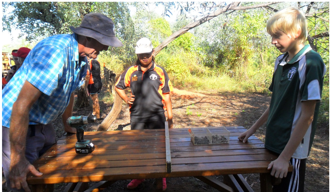
Unit Leader Huby Vink helps the Bush Rangers install a newly made picnic bench
