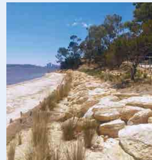
Riverbank foreshore restoration works were carried out at Point Heathcote in Applecross. Photo – DBCA
