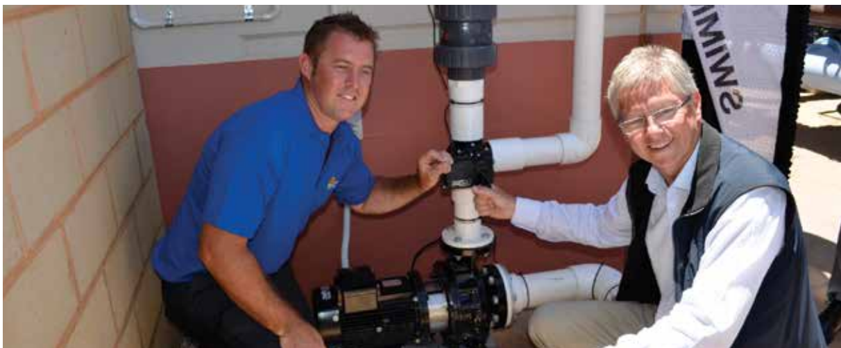
Environment Minister Bill Marmion switches on the solar thermal heating for the City of Kalgoorlie-Boulder's Goldfields Oasis Leisure Centre.
