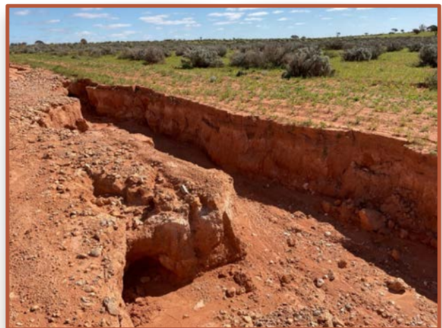
Track erosion due to March rainfall in the GVD. Photo: Pila Nguru Aboriginal Corporation
