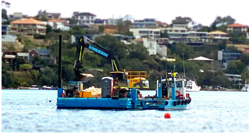
Installing limestone substrate at Point Walter in the Swan River. Photo credit: Tony Jupp
