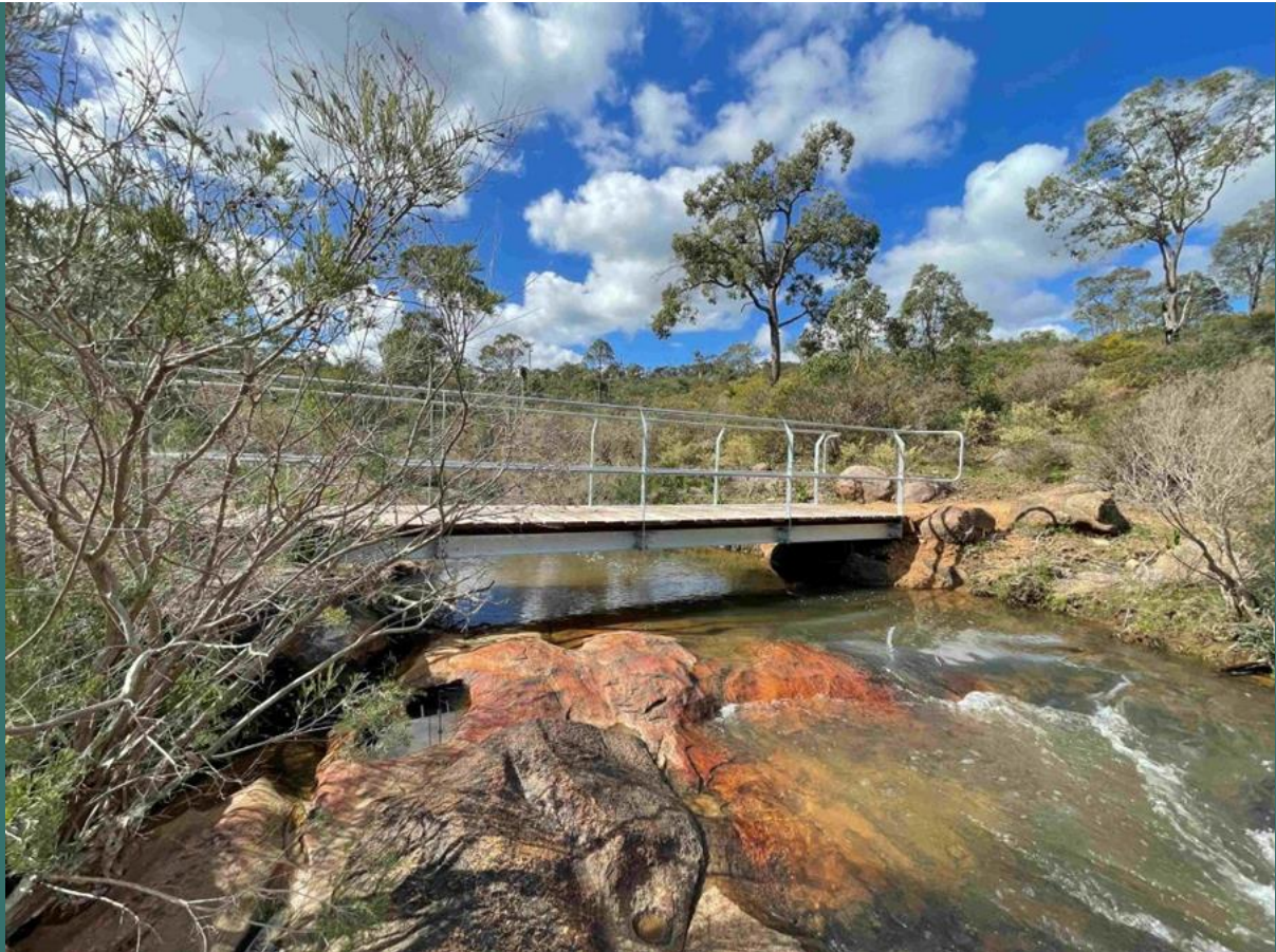
A bridge across Glen Brook. Credit: Jamie Wright/Department of Biodiversity, Conservation and Attractions
