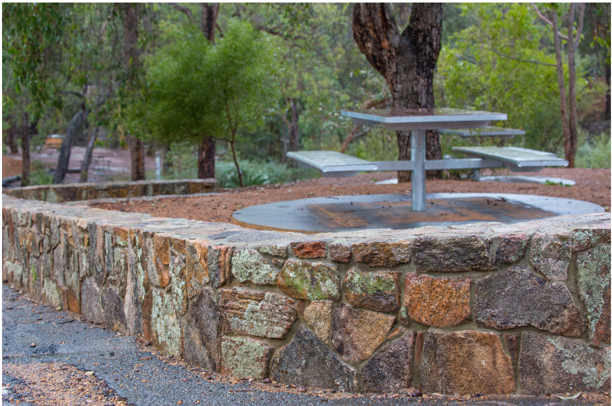
Reconstructed walls and new picnic facilities at John Forrest National Park (Photo: L-A Shibish)
