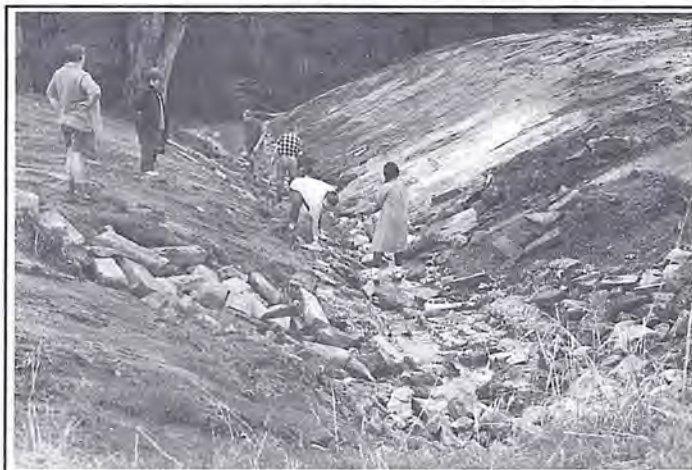
Clearing work after volunteers relocate rubble to reduce water flow at the Southernwood Creek site. Matting to reduce erosion and tree planting has since been undertaken.
