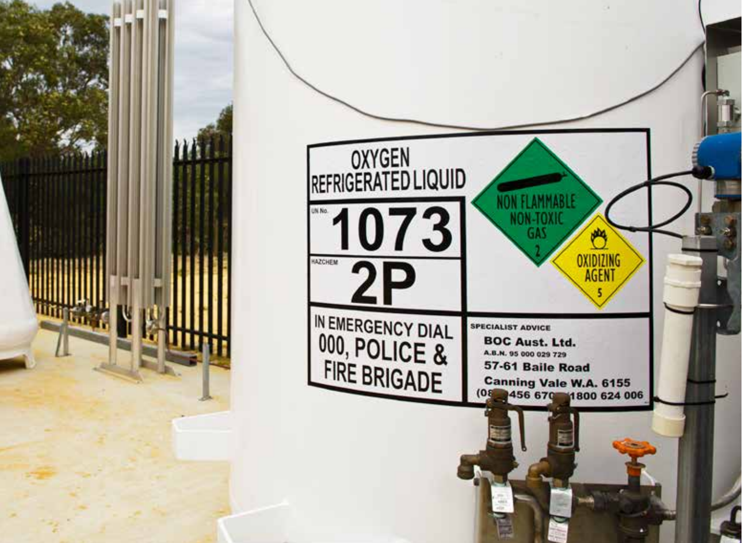
A new oxygenation plant at Nicholson Road Bridge on the Canning River will come online this year. Page 15: Swan River Trust river health program manager Alex Hams at the Bacon Street plant on the Canning River. Pictures: Stewart Allen.
