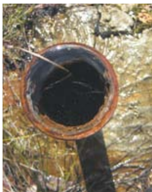
Groundwater overflowing from monitoring bore in Cobiac catchment.
