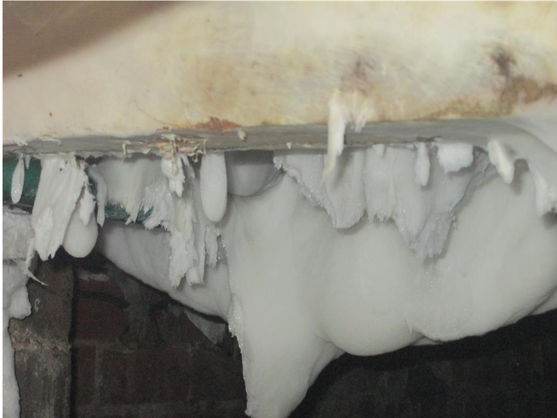
Figure 16: Damage caused by Serpula lacrymans infestation
