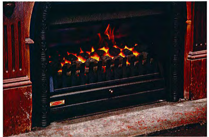
A flued gas heater
