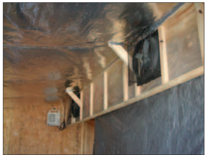
Figure 2—An electric heater in rear of solar dry kiln. Note lack of aluminum foil insulation on the sidewall showing the uncovered structural insulated panels (SIPs).
