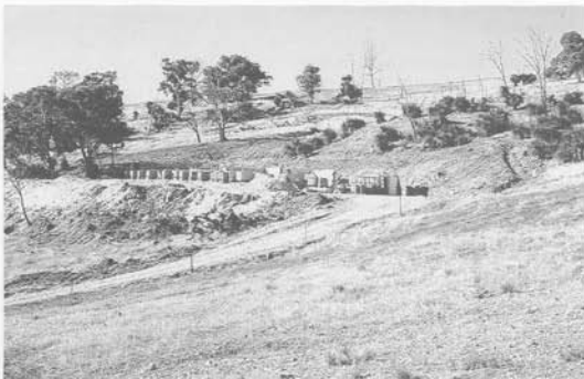
House construction using a concrete slab foundation. The amount of excavation required to provide a level site is determined by the slope gradient.
