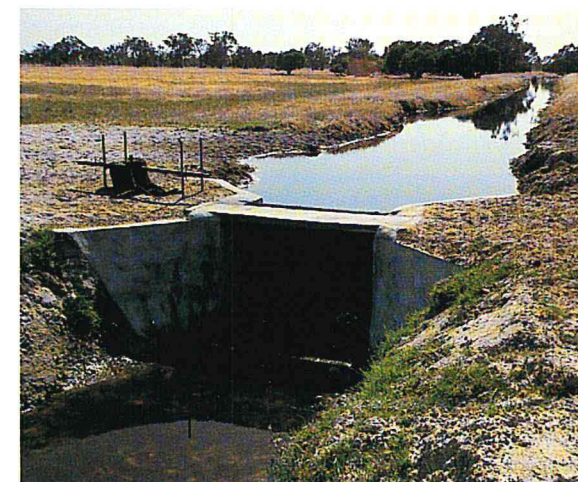
Water retention structure (lock) built on the Mealup Drain to better manage the drainage in the area
