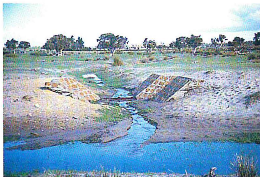
An unprotected feeder drain entry point
