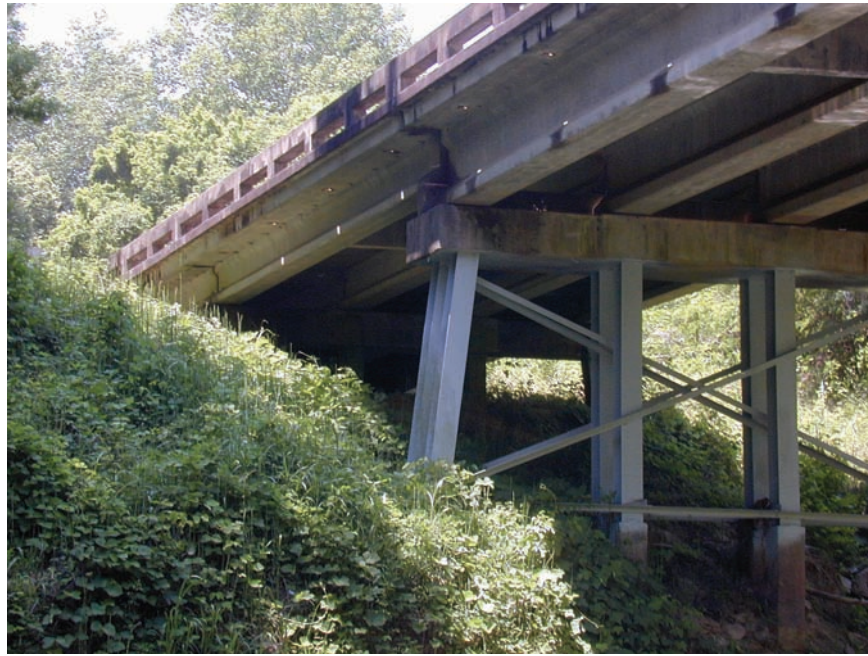
Figure 2—Concrete girder bridge in Claiborne County, MS, used as a maternity roost by > 30 Rafinesque's big-eared bats in 2009. (Photo by Monica Wolters)
