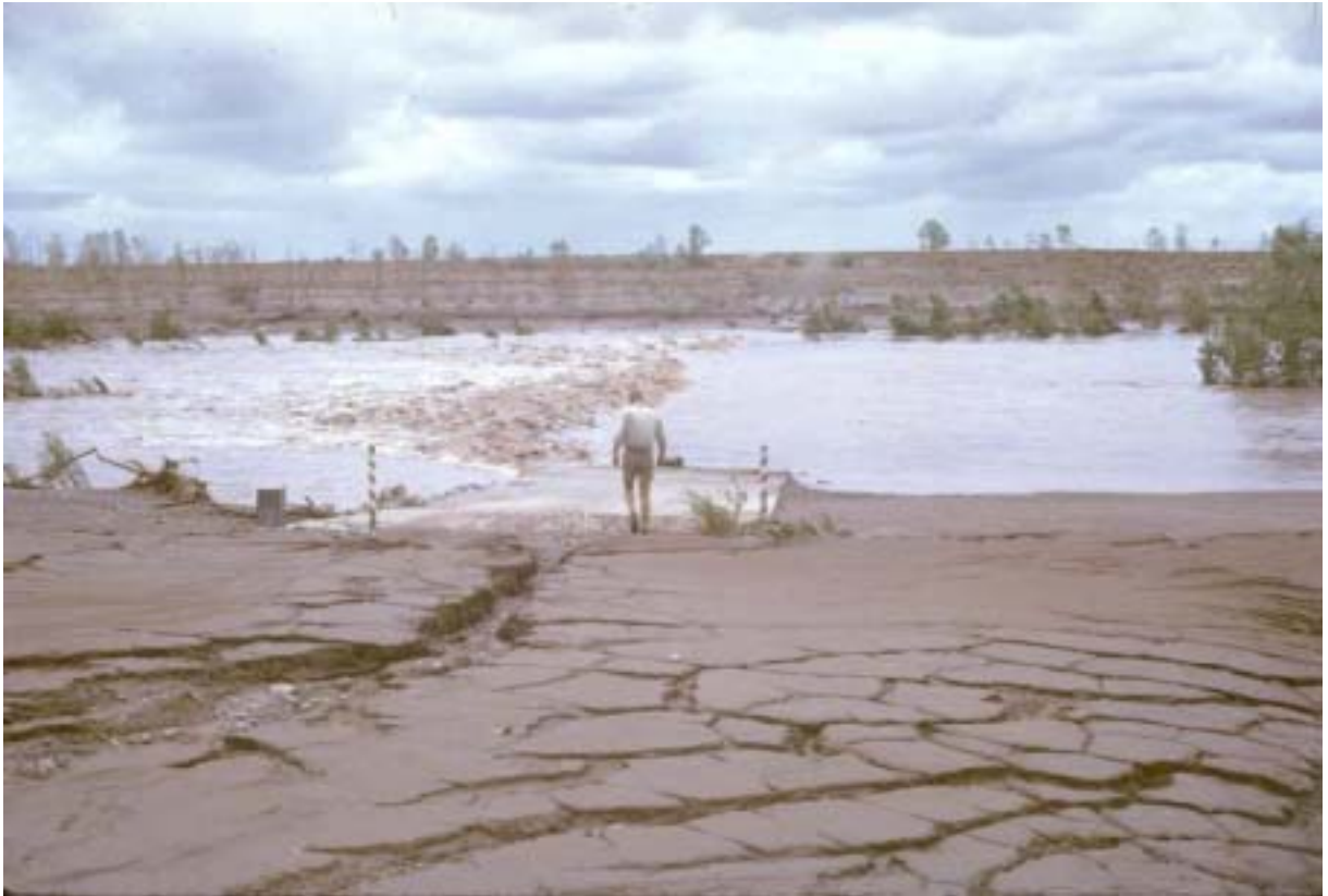
Photo 33. Duncan Road crossing on the Negri River showing large amounts of sediment deposited on the crossing by the river. May 1963.
