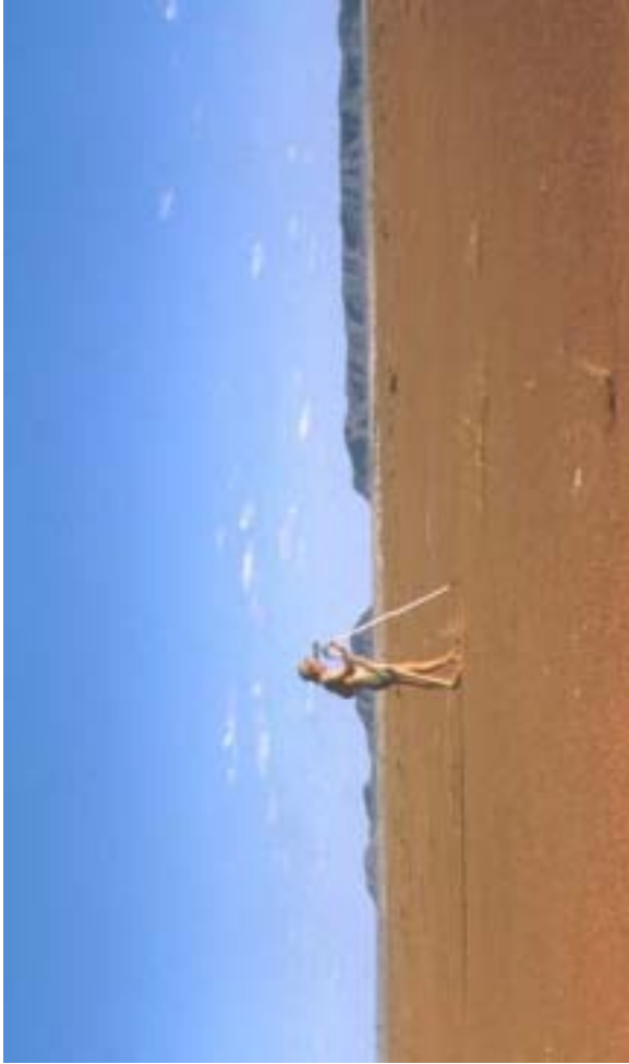
Photo 37. Contouring with a dumpy level for strip cultivation works on the Turner Plains. June 1960.
