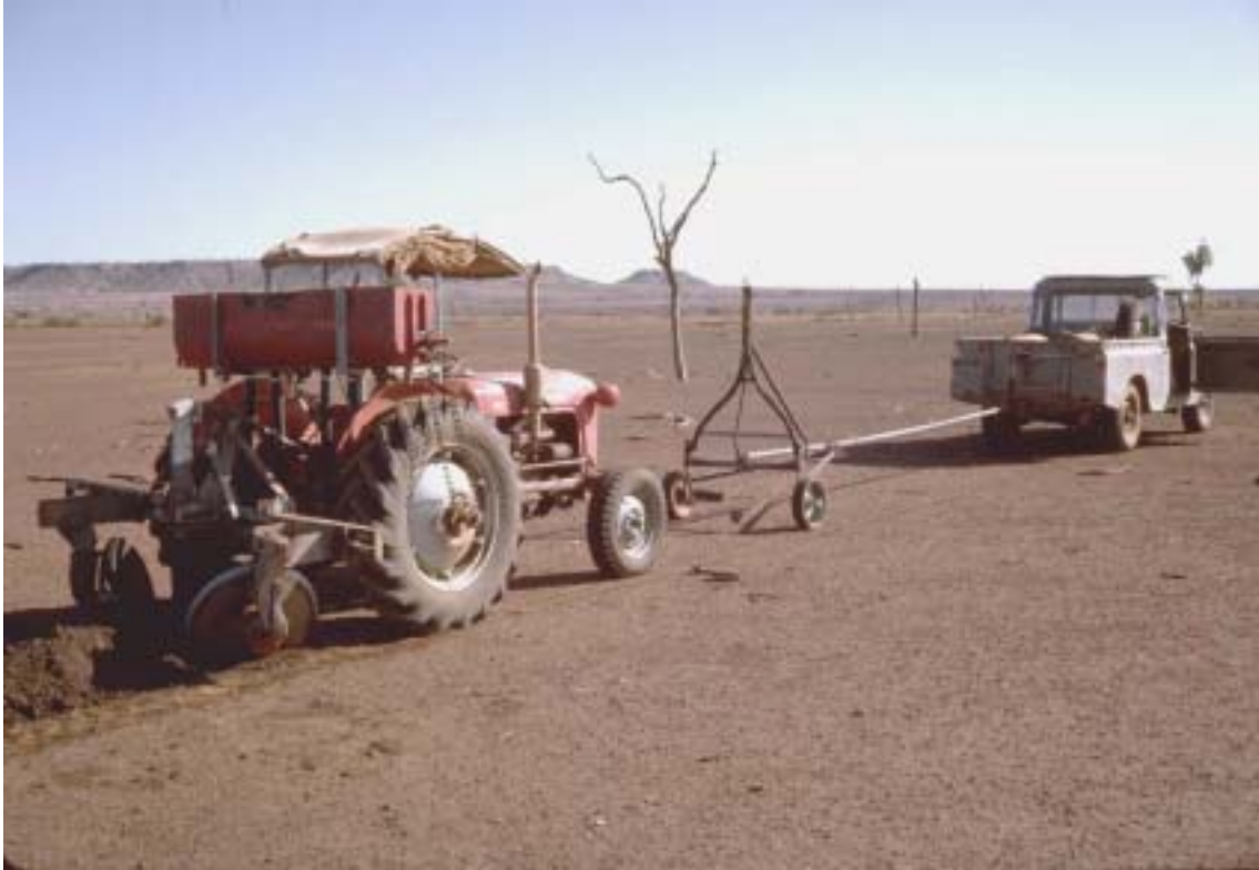
Photo 13. A tractor equipped with a twin opposed disc plough and centrally mounted ripper is following a mobile hose level which is marking the contour line. June 1964.
