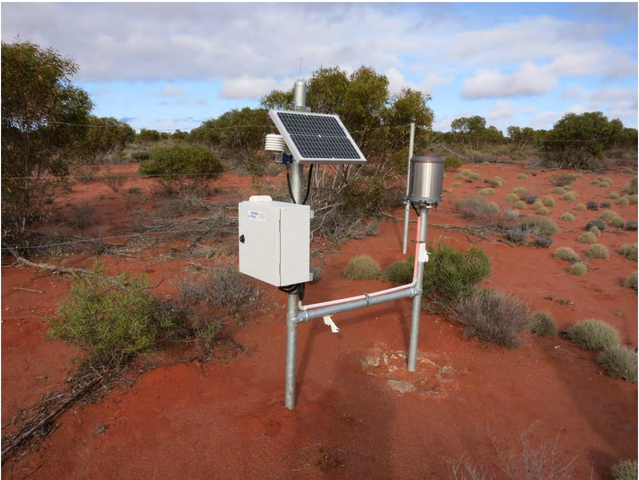
Figure 3 Installed weather station
