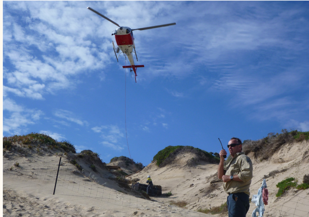
A helicopter brings in materials for the coastal rehabilitation project at Ellensbrook and Prevelly.
