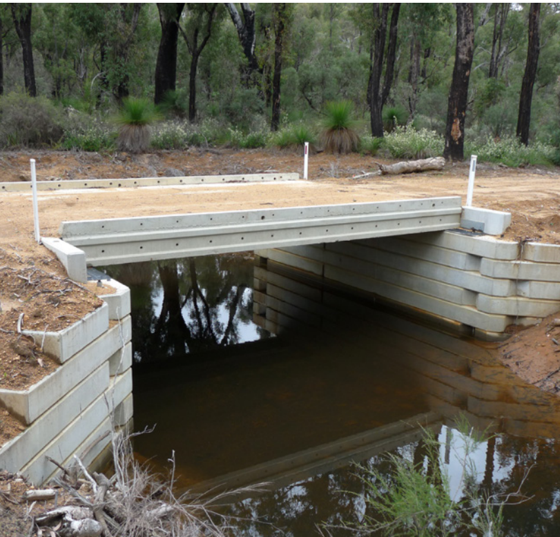
The department's new concrete modular bridge is stronger and lasts longer than the existing timber bridges. Photo – Mark Graves/Parks and Wildlife
