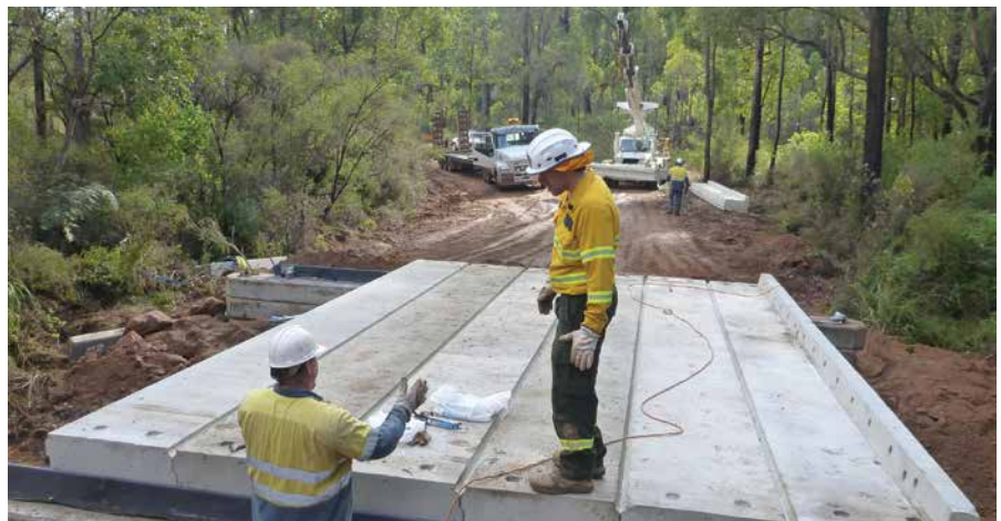
Phil Griffiths and Tim Hutton building Scarp Road Bridge at Logue Brook Dam. Photo – Carl House
