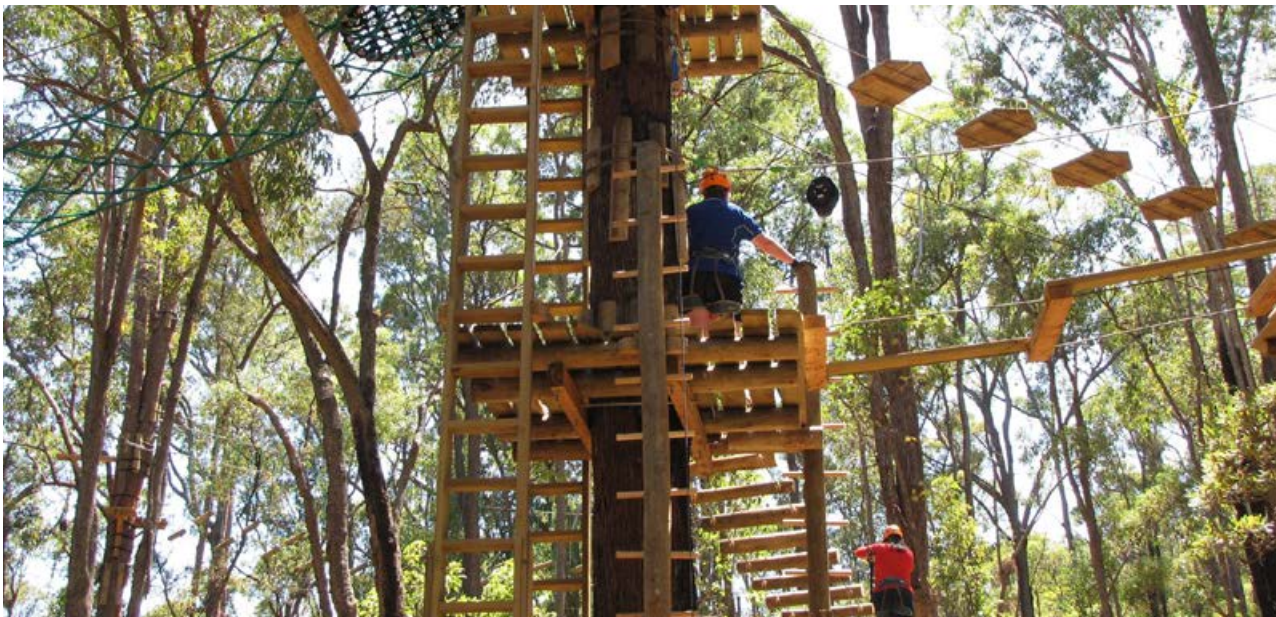
Obstacles are built around trees to minimise impact, with timber clamped to the trees rather than drilled into them. Photo – Lauren Emmerson/Parks and Wildlife
