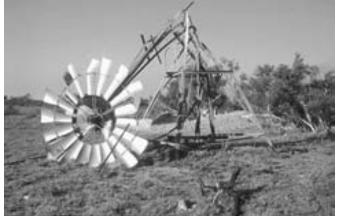
Damage to infrastructure, such as this windmill, caused by cyclonic winds is an annual risk.
