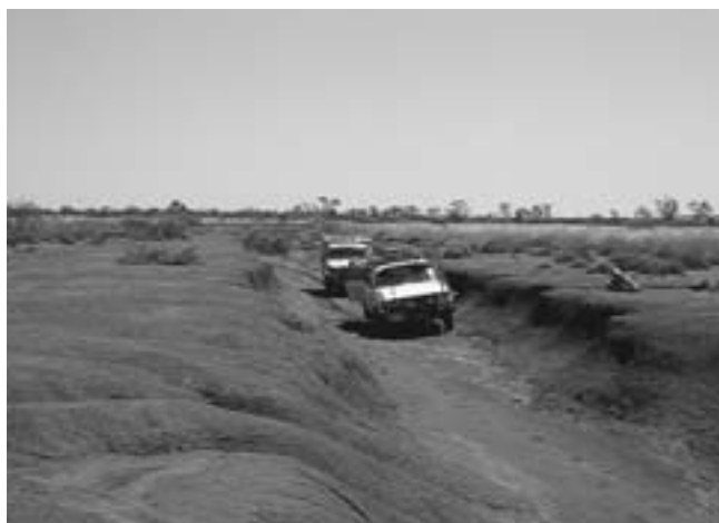
Inappropriately located tracks can lead to erosion. This former track is now effectively a channel for diverting overland water flow away from other areas.
